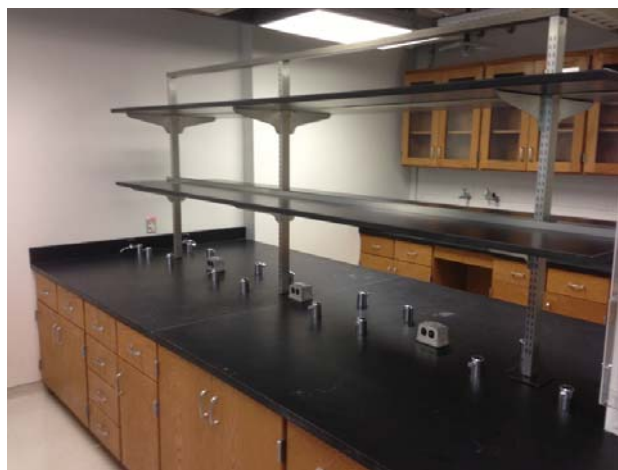
Can be used in retrofits of existing labs
